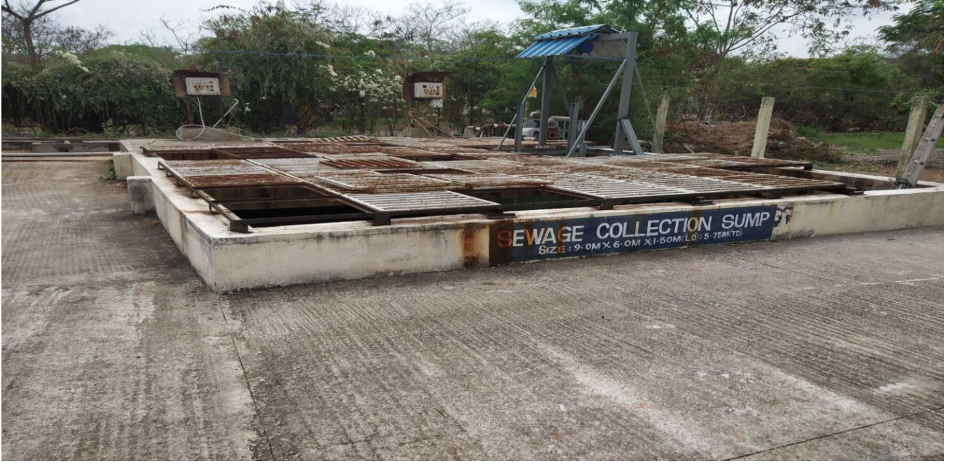
Sewage Collection Tank
