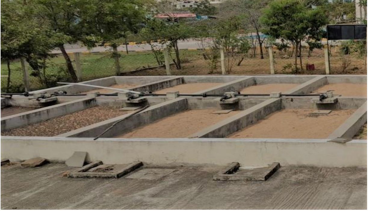
Sludge Drying Beds -8 Numbers (4 Nos on each side)
