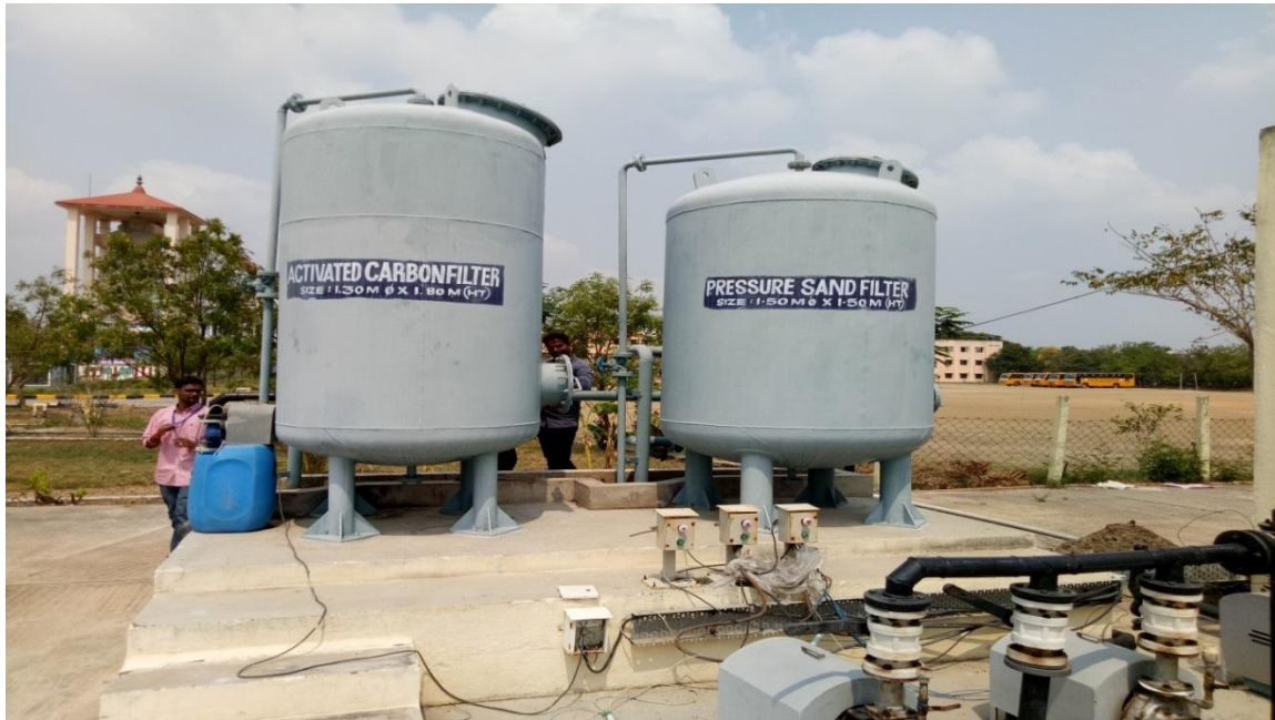
Pressure sand filter Activated Carbon filter
